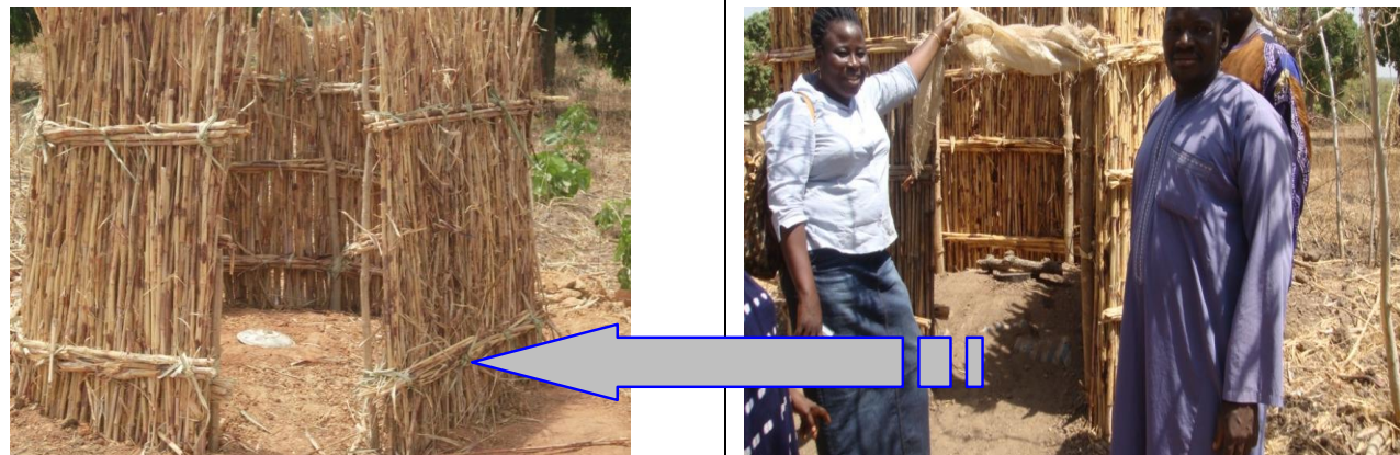
Sanitary facility built by a community member
